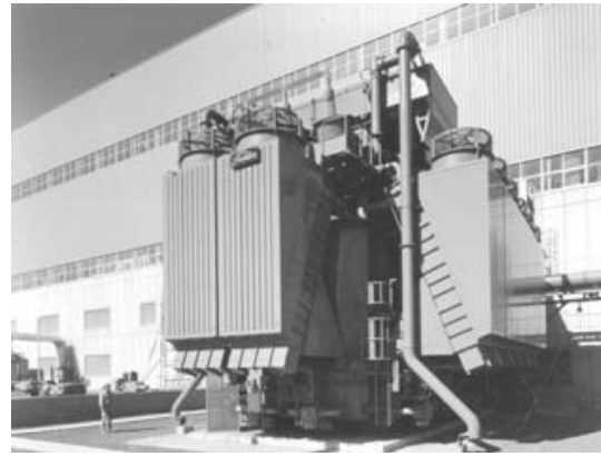
Photo 4.13. An 1100MVA Transformer for the Tokyo Electric Power Company Kashima Power Station (1973, made by Toshiba)
