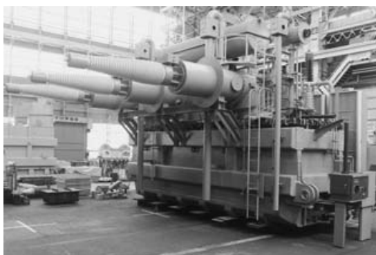
Photo 5.18. A 250kV DC Transmission Transformer at the Electric Power Development Company Hakodate Converter Station (1979, made by Hitachi)
