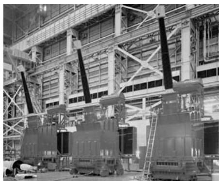
Photo 5.2. The First 765kV Transformer, an 805/3MVA Transformer for Venezuela (1982, made by Mitsubishi)
