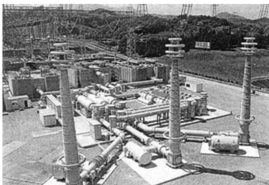
Photo 5.16. UHV Demonstration Testing Transformer at the Tokyo Electric Power Company Shin-Haruna Substation (1993, from left made by Toshiba, Mitsubishi and Hitachi)
