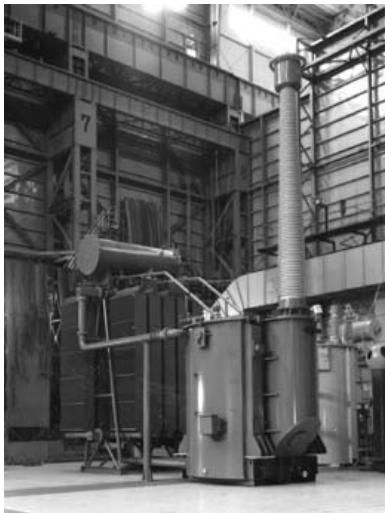
Photo 5.7. A 765kV, 400/3MVA Shunt Reactor for South Africa (1985, made by Toshiba)
