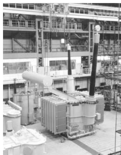
Photo 5.3. A 765/500kV, 1650/3MVA Transformer for Brazil (1988, made by Toshiba)
