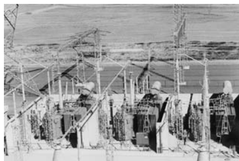
Photo 5.4. A 765kV, 2000/3MVA Transformer for South Africa (1985, made by Fuji)
