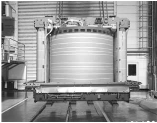
Photo 5.14. Interior of the Higashi-Shinjuku Substation Transformer
