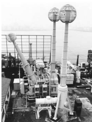
Photo 5.1. UHV Prototype Transformer (1979, made by Toshiba)
